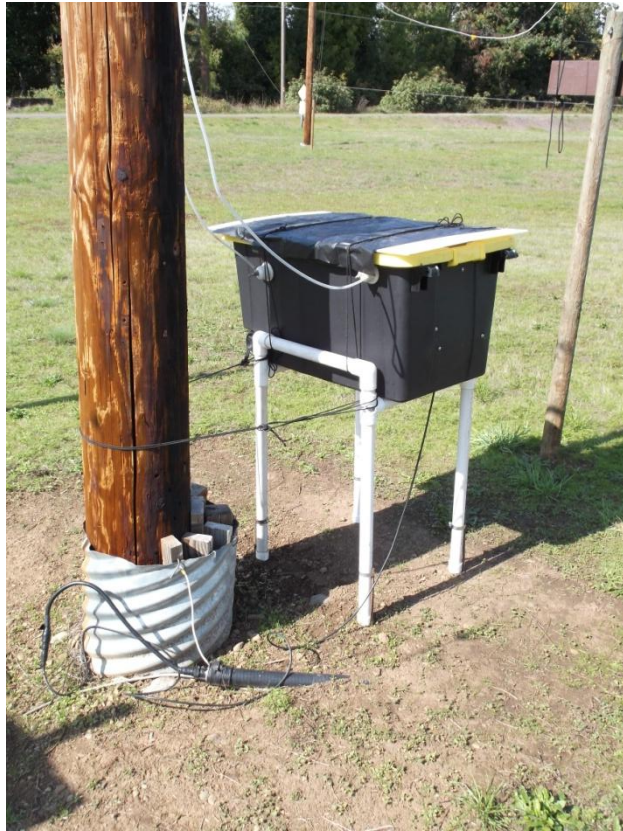
Figure 10 - 2200m tuner installed.
